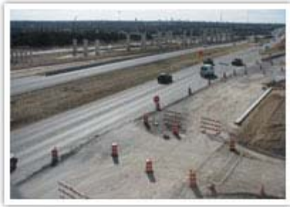
Footings and columns are placed for the direct connect flyovers at US 183.
