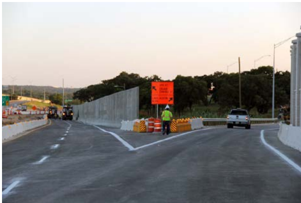
Crews striping the temporary SB Cesar Chavez/5 th St./Lake Austin Blvd. exit as they prepare to open it.
