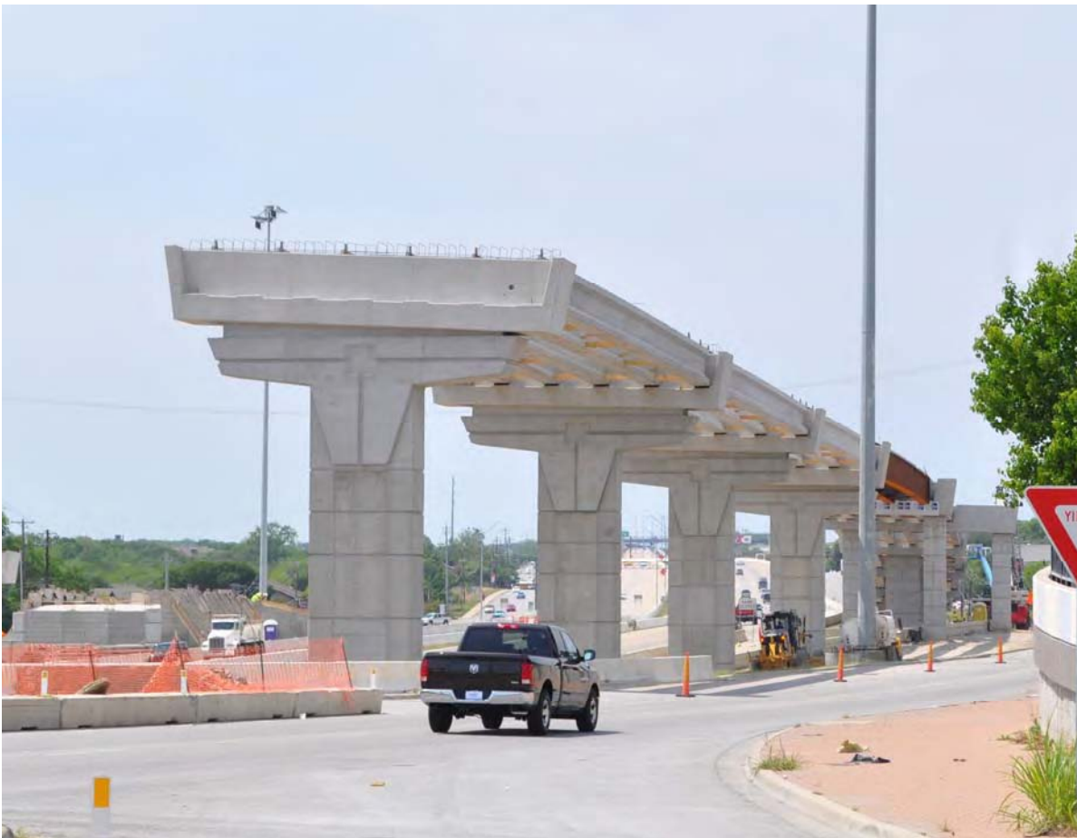
Ongoing construction work at the west to north direct connector [taken April 13, 2011]
